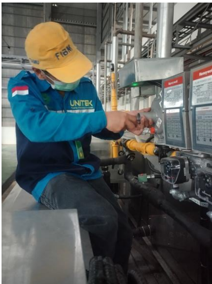
Service maintenance & calibration
